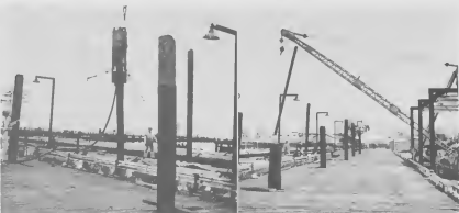
THE TRESTLE that once supported the rails for sulphur carrying carts will soon be dismantled. It will be replaced by a six-foot-wide walkway to the Gasoline Docks. Until 1954, Lago imported its sulphur requirements from Louisiana.
